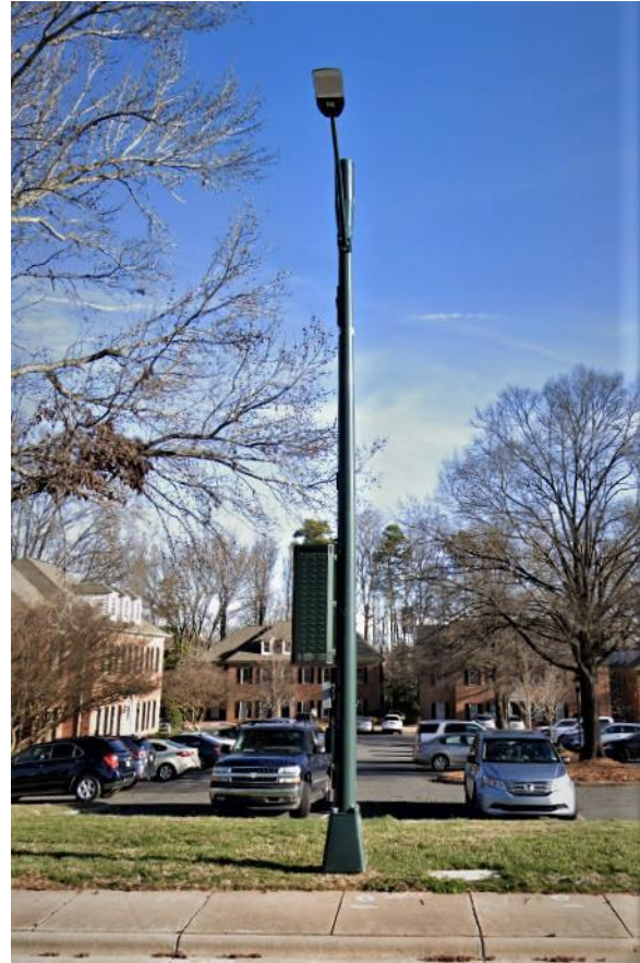
"Dual Use" utility-owned pole with 4G small cell in Charlotte
